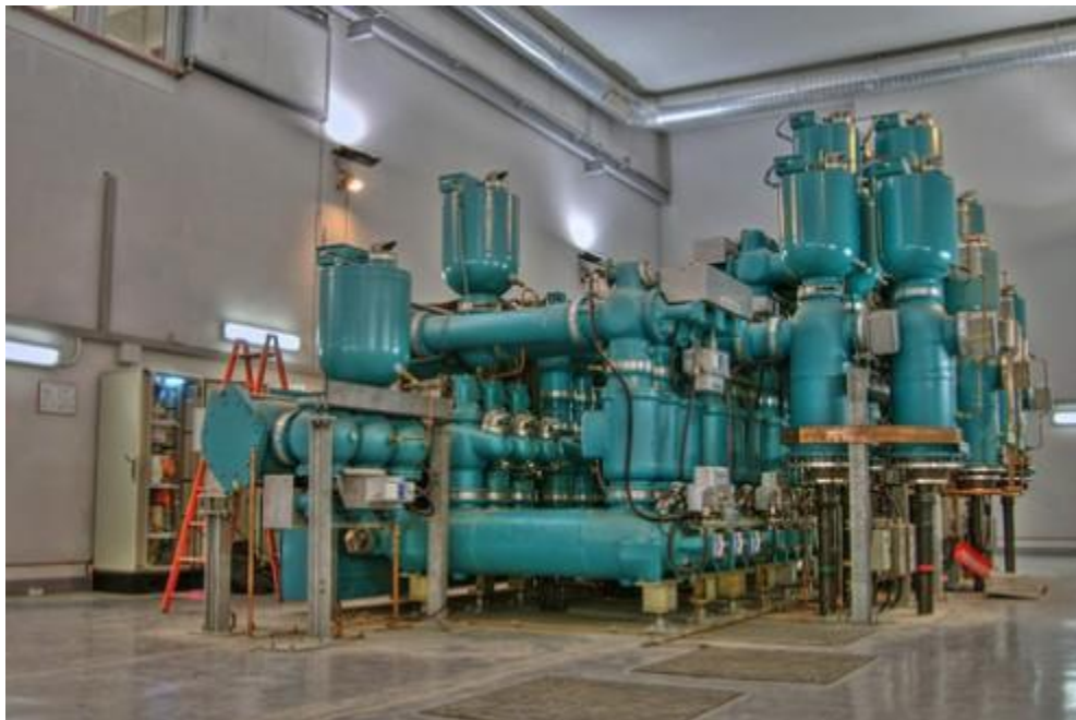
Gas Insulated Substation
